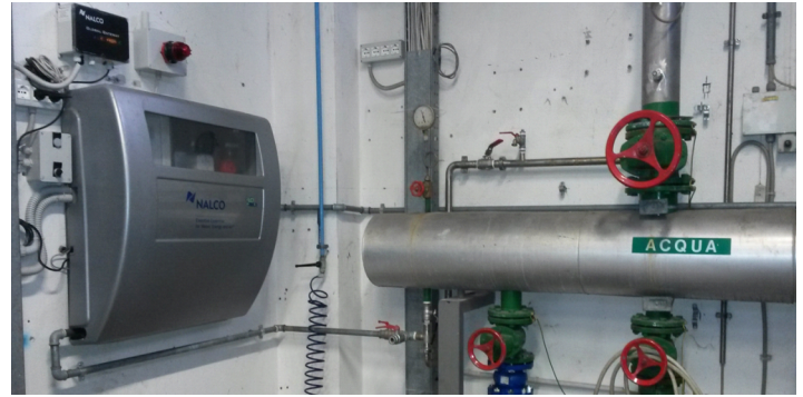
Nalco Water 3D TRASAR unit in the retorts cooling system
