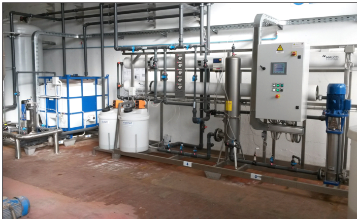
The new Nalco Water RO plant
